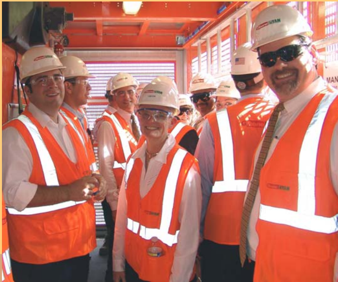
A group of administrators and Judges climb aboard a construction elevator on the south side of the Criminal Court Tower.
