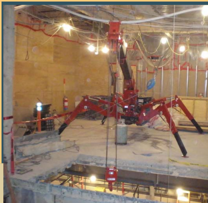
The Spider Crane is helping with steel construction on the Central Court Building Escalator Project.
