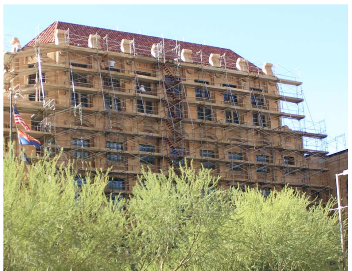
The Old Courthouse is getting an updated look. The majority of the renovation centers around new windows.
