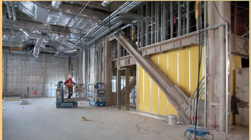
An inside view of the progress made on the Criminal Court Tower.
